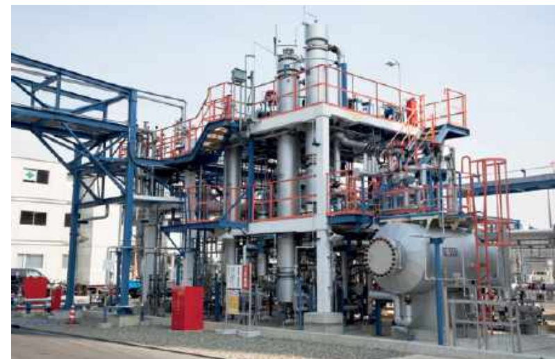
01 Dehydrogenation plant reaction area. Source: Advanced Hydrogen Energy Chain Association for Technology Development
