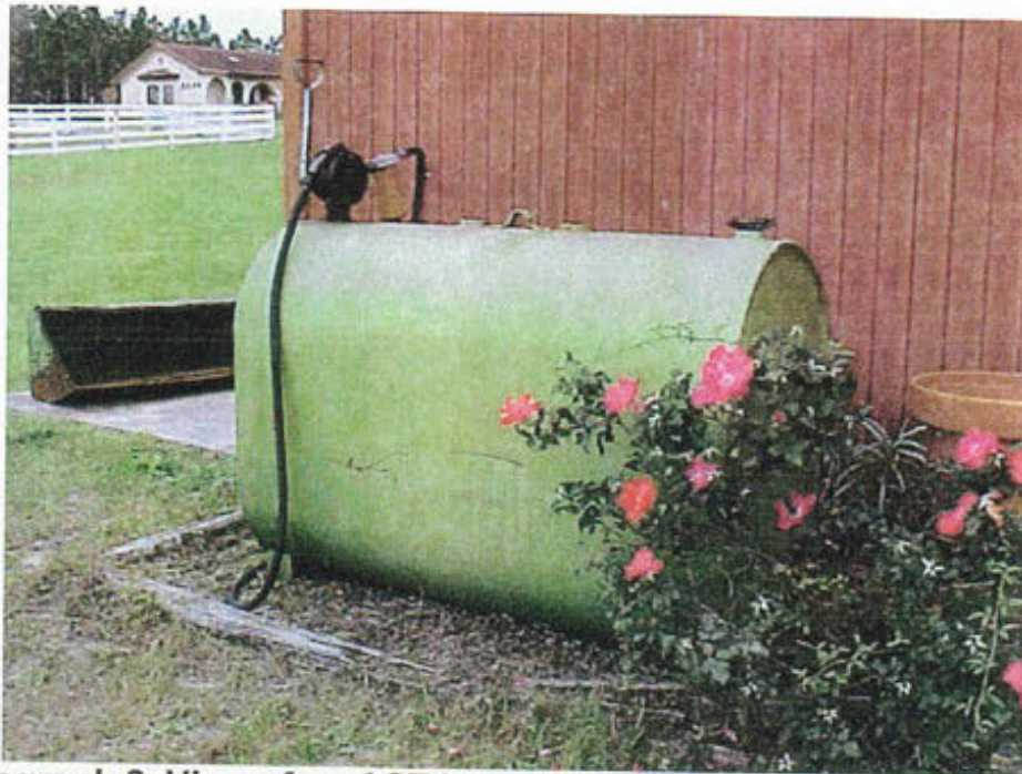
Photograph 8. View of an AST located on the southeast portion of the subject property
