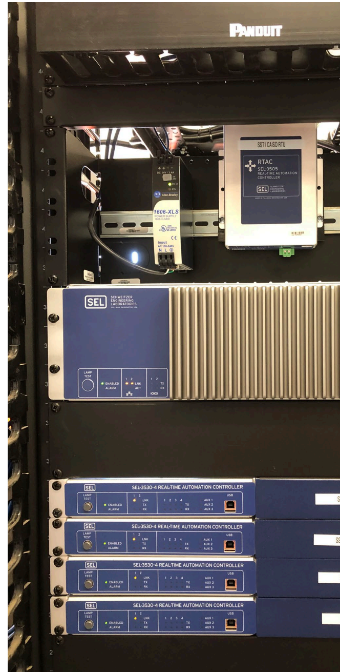
POWER PLANT CONTROLLER CABINET
