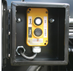
Lifting and lowering control buttons inside steel box.
