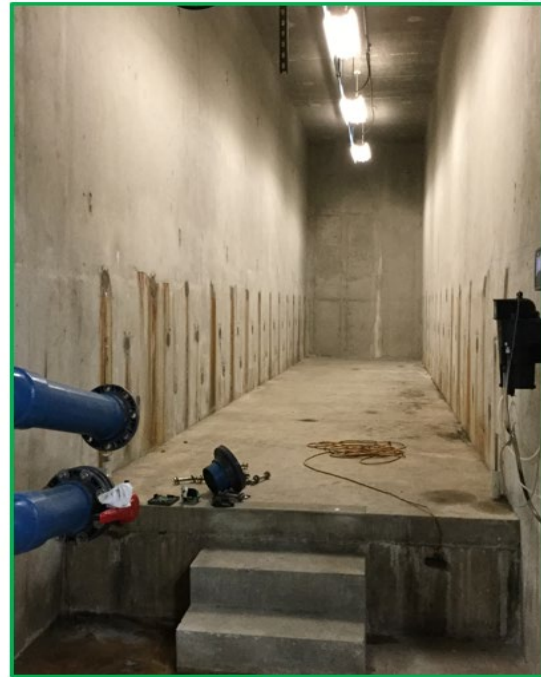
After Removal of redundant piping, valving and actuators not needed with FibrePlate operation
