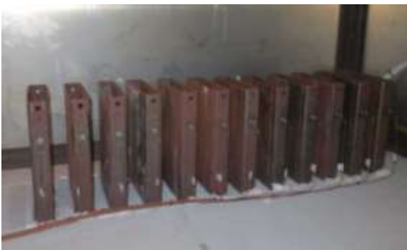
Surface corrosion on riser ducts as seen from within outlet plenum
