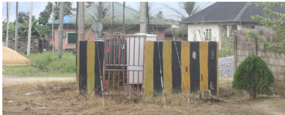
Allegedly used transformer, installed for Ekpetiama Clan
