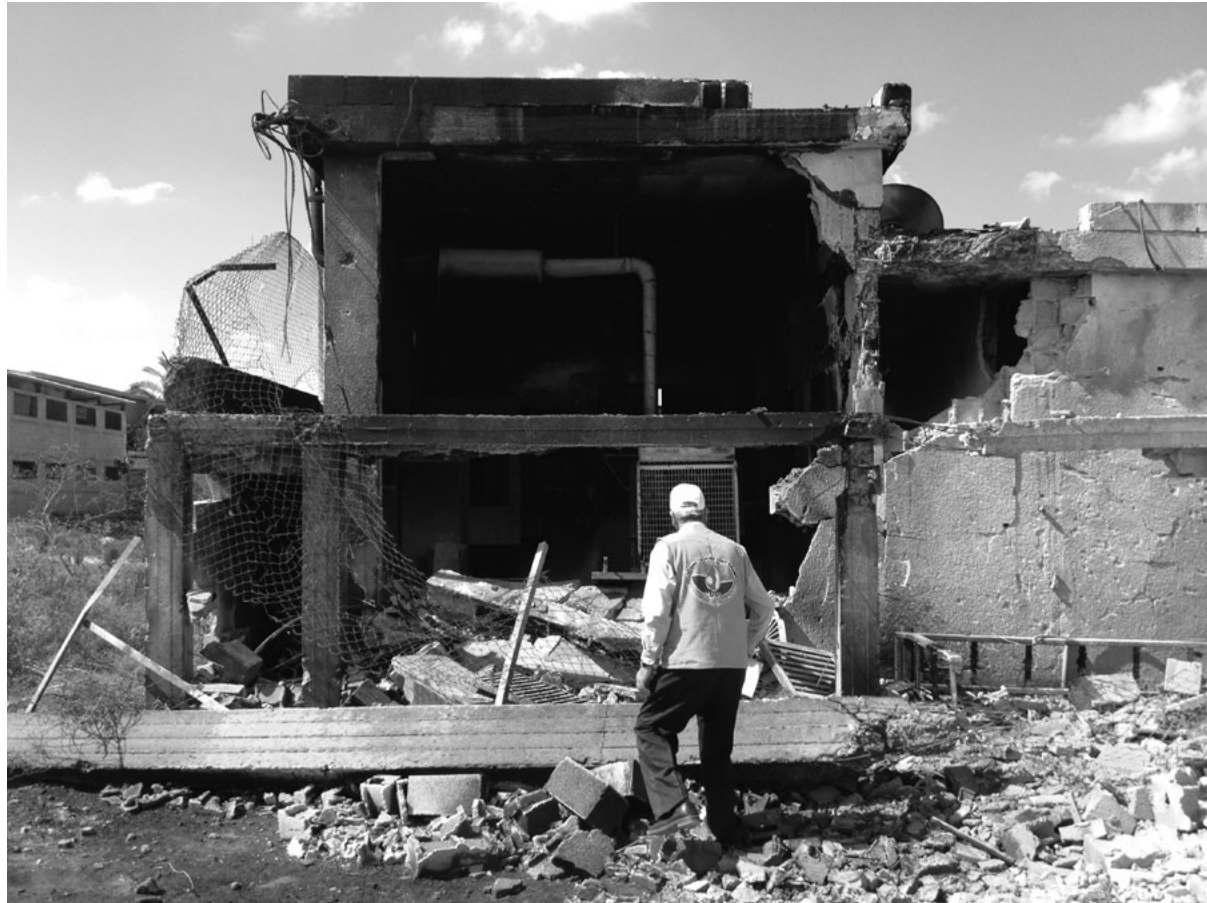
An engineer from the Coastal Municipalities Water Utility inspects a damaged sewage pumping station in Beit Hanoun, a high density urban area close to Gaza City.
