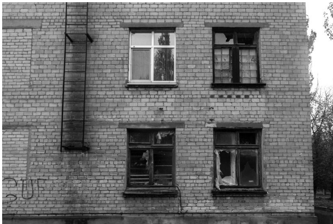
Explosive weapons caused broken windows at Maryinka District Central Hospital.
