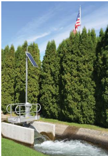
Each FlumeGate's responses are tailored to the channel they are regulating
