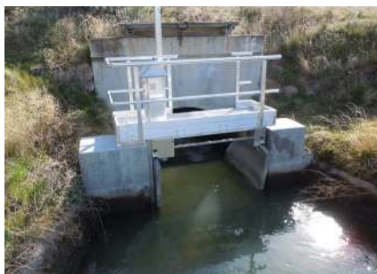
Network Control performs well in hydraulically challenging environments
