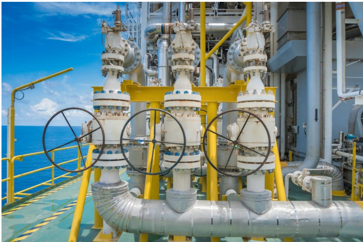
Set of 3 PSV's and 3 inlet block valves
