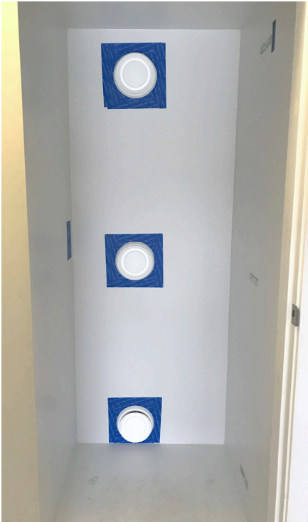
Figure 9 - Air Sealed Chamber and Exhaust Diffusers
