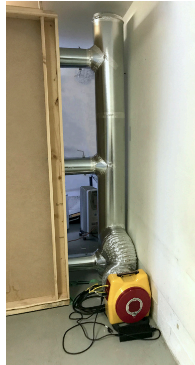
Figure 10 - Measurement Fan and Ventilation Trunk
