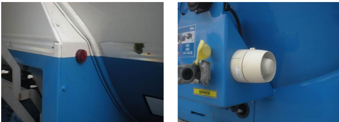
Figures B-3 Visual and acoustic warning signs
