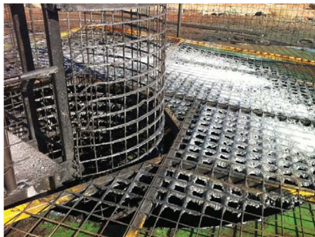
FIG 1 - Installing a ladderway in a surface exhaust is very poor practice.
