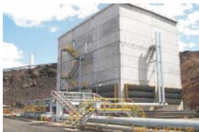
FIG 7 - Surface bulk air cooler (photo courtesy of Mount Isa Mines Limited). BAC is 22 m high × 16 m deep × 24 m wide, and is capable of cooling 750 kg/s of intake air from 25° C WB/43° DB to 14.1° C WB/DB.
