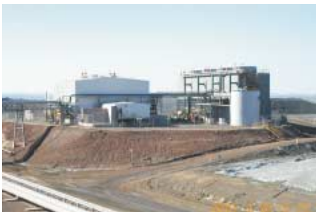
FIG 6 - Surface refrigeration plant and condenser cooling tower (photo courtesy of Mount Isa Mines Limited). The refrigeration plant is to the left with the condenser cooling tower to the right. Plant capacity is 25 MW(R).
