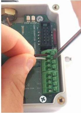
Second wire connection
