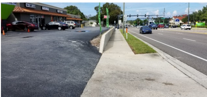
Figure 10: Steep driveway and sidewalk cross slopes
