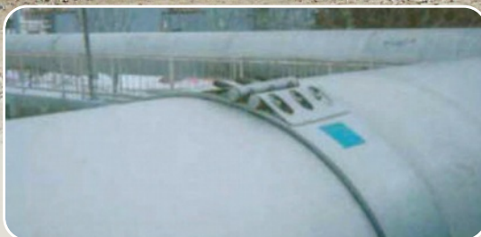
▲ 48" (1,200A) YNMF-RL Canadian power plant cooling line
