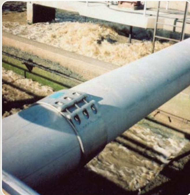
▲ Spain: water purification facilities
