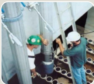
▲ Canada: water purification facility
