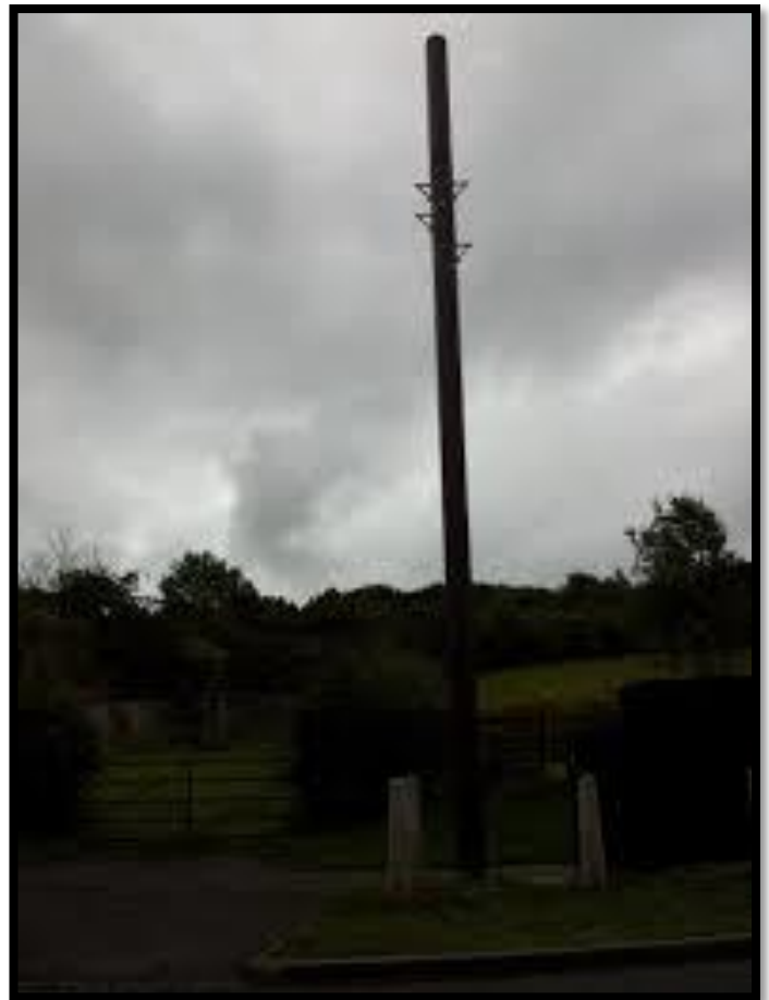
Figure 5 Example of a telegraph pole slim design supporting antennas in a rural area
