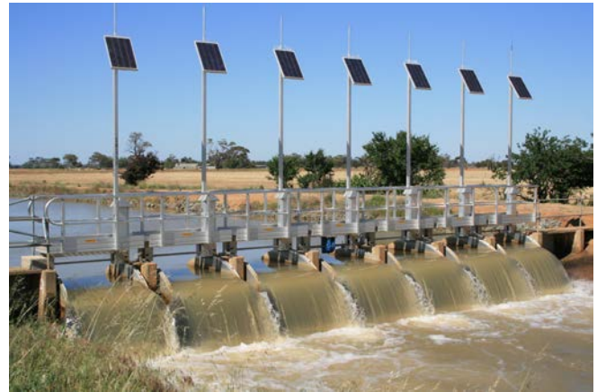
Automated gates installed on a channel as part of the Connections Project.
