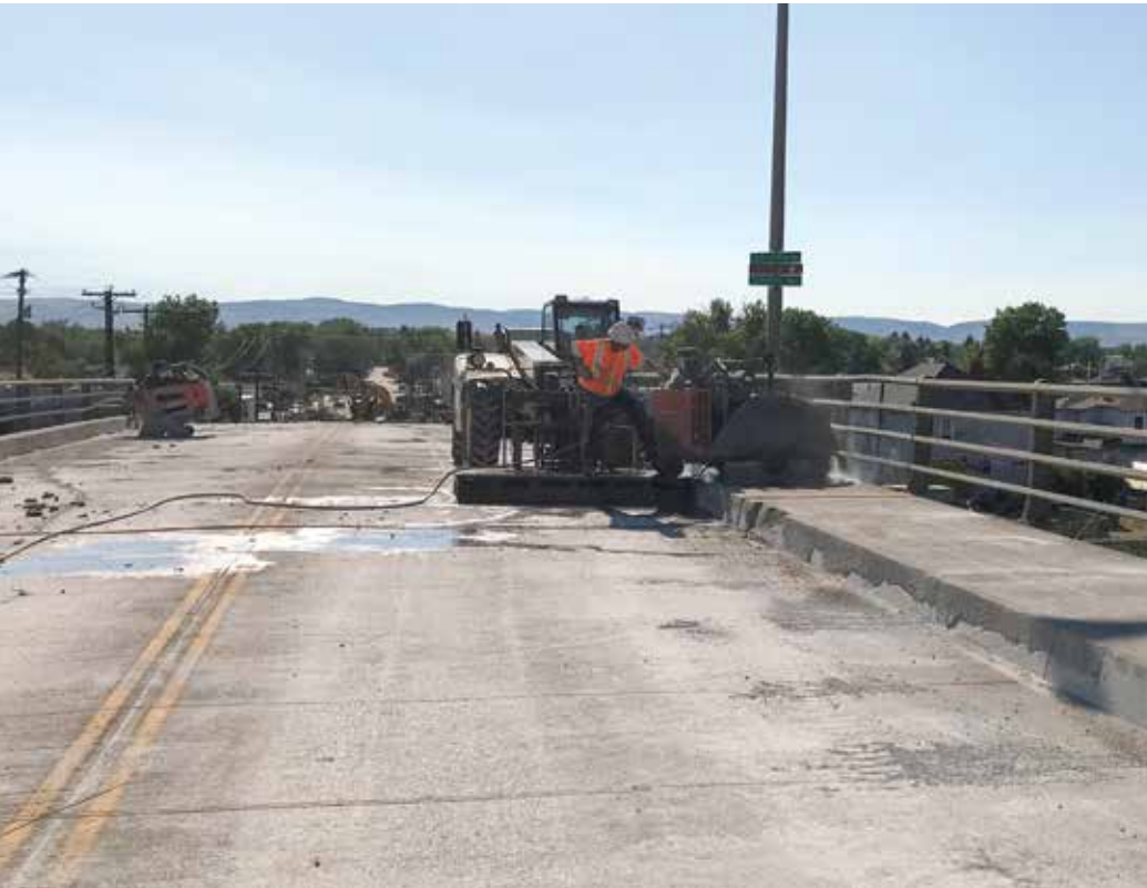
Husqvarna slab saws with up to 36" blades were used to cut the bridge deck into 14-foot by 6-foot sections.
