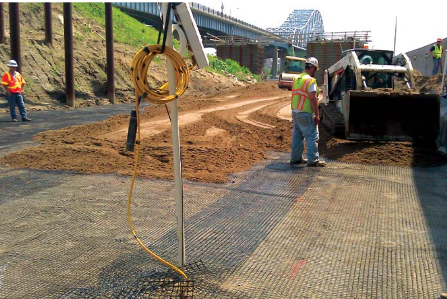
FIGURE 4 A layer of geogrid reinforcement is backfilled with fine sand to create the LTP for the new Hastings bridge approach.
