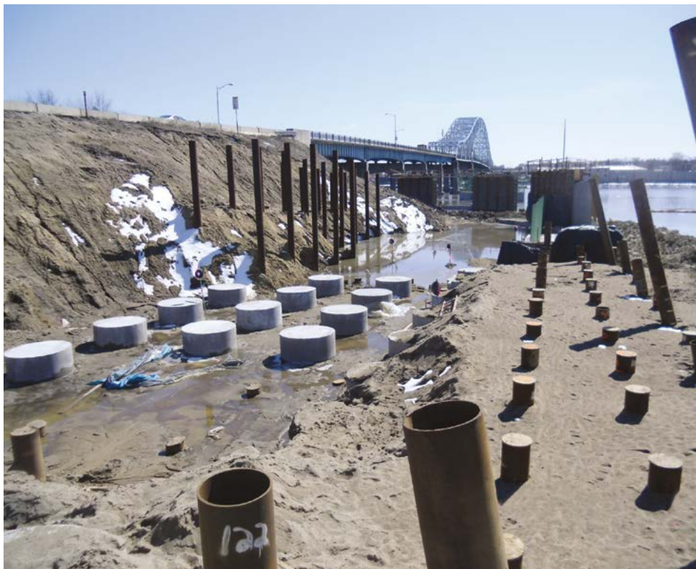
FIGURE 3 Some of the concrete pile caps (left side of photograph) and concrete filled pipe piles driven (right side of photograph) before construction of the LTP for the new bridge.
