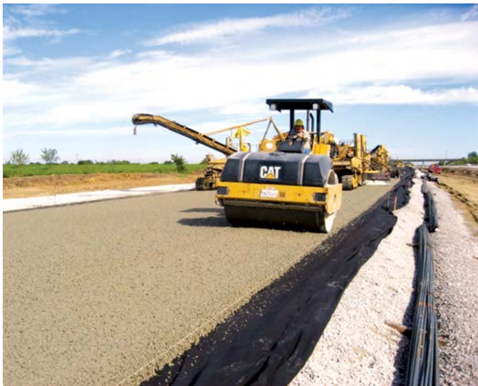
FIGURE 5 The CRCP rolled and overlaying the nonwoven geotextile separator and the geomembrane that provides the moisture barrier.
