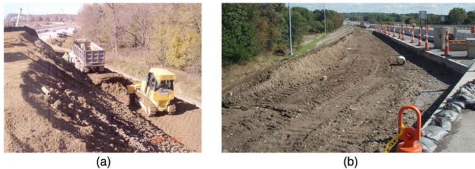
Fig. 4. Construction of sliver fill for lane widening on I-71 Southbound between Stations 420 + 80 and 421 + 80 LT looking (a) southbound with I-76 in the foreground; photograph used with permission from Ruhlin Company; (b) northbound along I-71 (photograph used with permission from ODOT)
