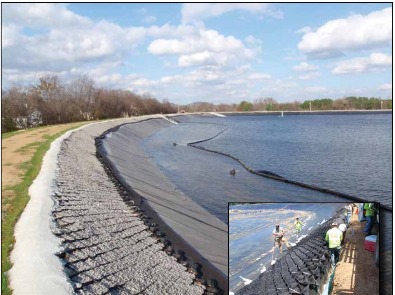
Completed reservoir rehabilitation shown now full of water. Inset: Installation of geoweb along the side slopes.
