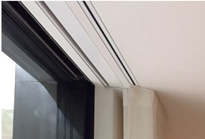
RT1F with SG51MB1F and SG51RB1F, installed in front of box.
