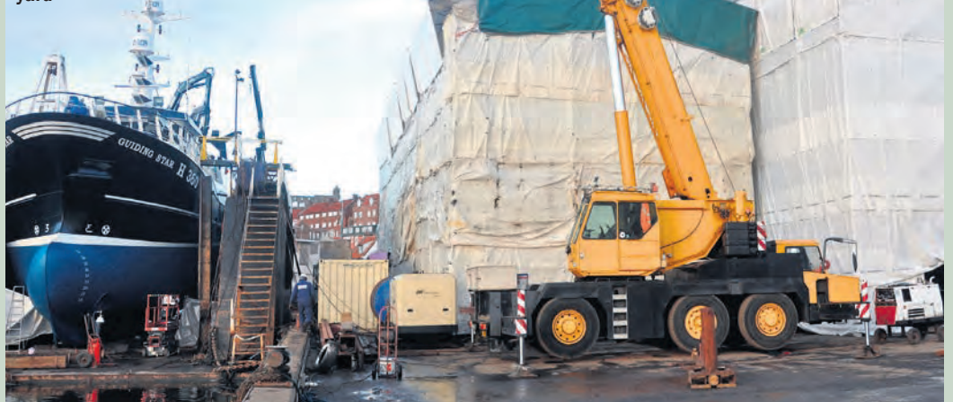
Guiding Star on Parkol floating dock last week while fitting out and machinery installation of another two new boats of similar size continues at the yard
